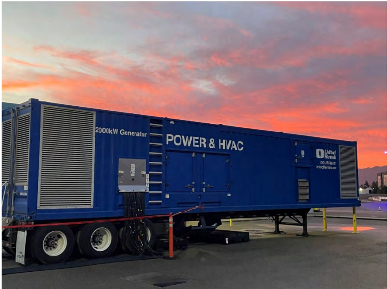
Photo: LAVWMA Rental Emergency Generator, January 12, 2023
